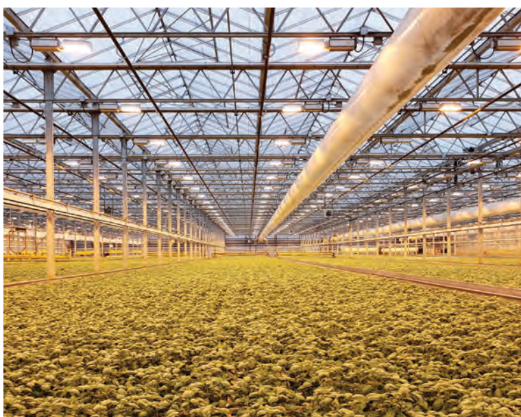
Figure 1. High-pressure sodium fixtures need periodic maintenance to achieve peak performance.
